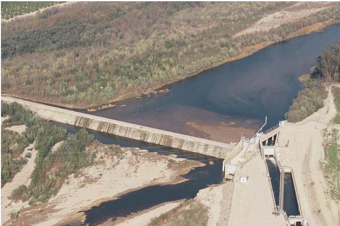
The Vern Freeman Dam and its Passage Infrastructure Extending Away from the Dam's Face
